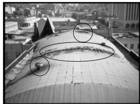
Defensive ventilation opening placed away from the seat of the fire. Example: Trench Cut
